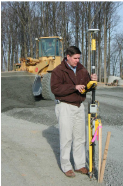
BC surveyor Evan Cregger using the Trimble 5700 GPS System as a roving unit to confirm a point during construction. The 5700 receives RTK corrections from an Air-Link Raven CDMA Modem.
