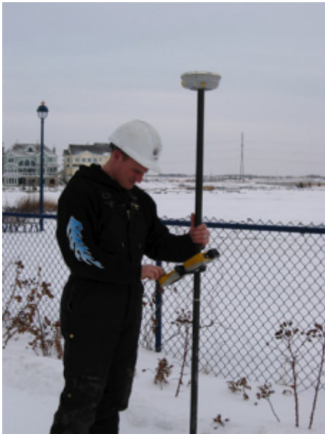
Stantec surveyor Trevor Pasika provides construction staking with the Trimble RTK GPS 5800 survey system on the Anthony Henday Drive road and bridge construction project in Edmonton, Alberta, Canada.
